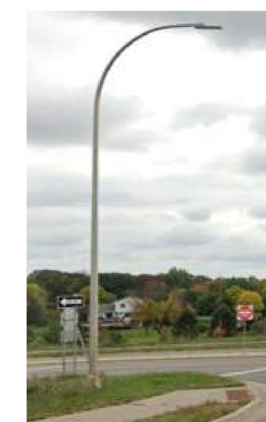
Lights at the roundabouts will match Armstrong Blvd lights
